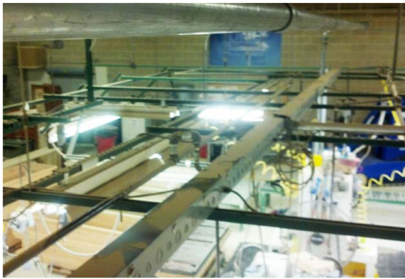
Wood dust covers the support structure beams.
